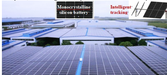
Figure 6 – Distributed Photovoltaic Power Generation System Installed on Plant Roof
