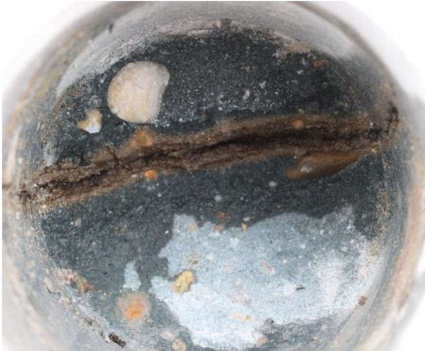
Crack in concrete substrate
